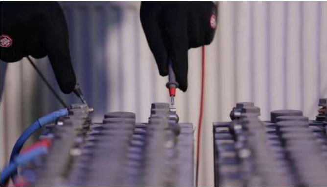
Capacity test on a stationary battery bank
