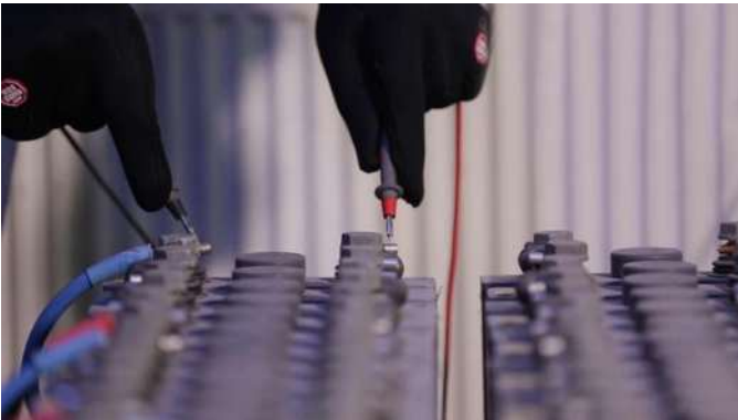
Capacity test on a stationary battery bank
