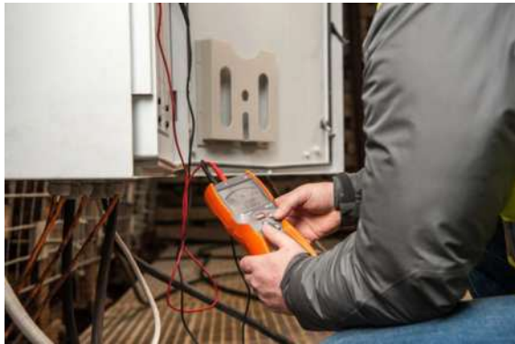
Continuity testing with the AMIC-30 inside a distribution cabinet
