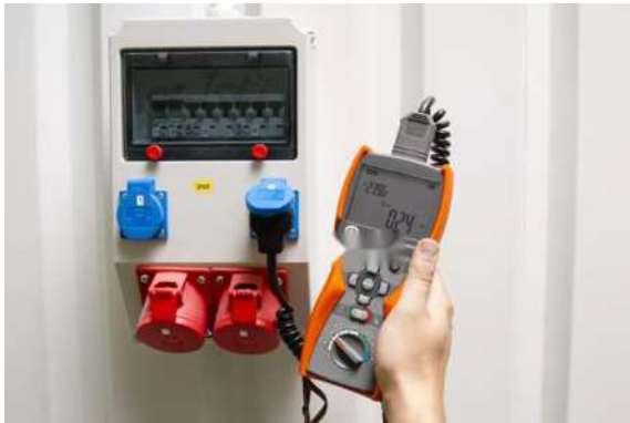
Loop measurement at an industrial board with the AMZC-304
