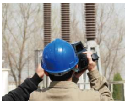
Substation survey with the installation in service
