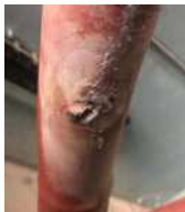
Field case: PD located on a cable termination
