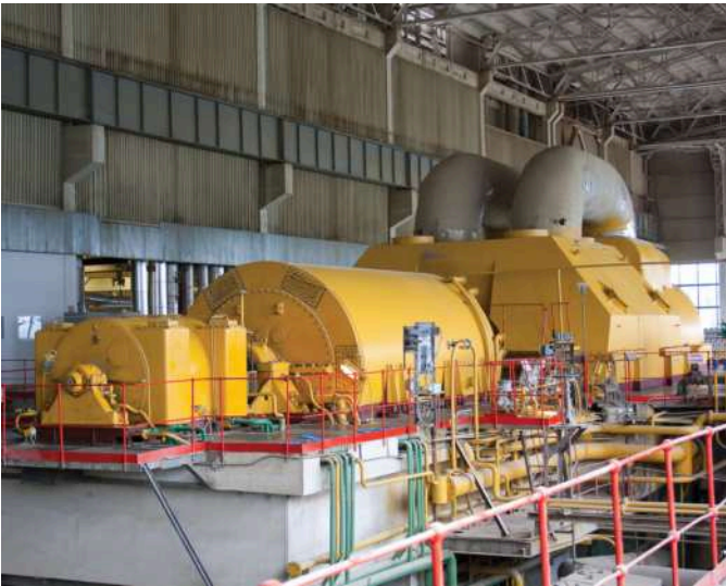
Turbo-generators and large motors: critical monitored assets
