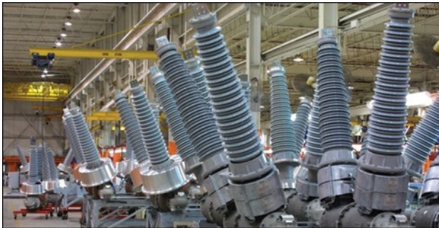
SF6 power circuit breakers.
