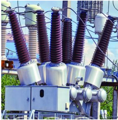
In-service high-voltage circuit breaker, showing the bushings and the operating mechanism where the BPM takes its measurements.
