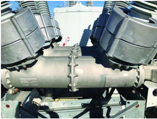
Operating mechanism and high-voltage circuit breaker, with the stored-energy system monitored by the BPM.
