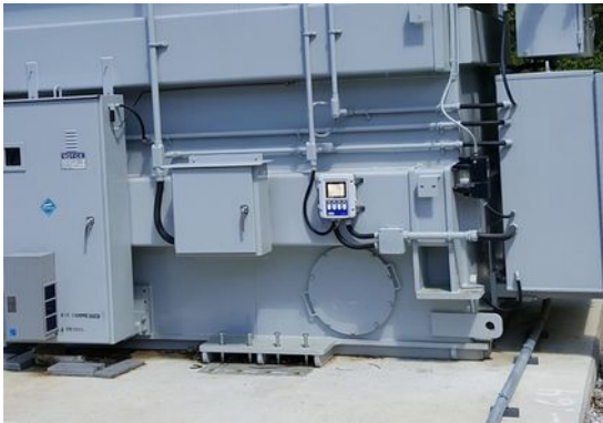
The B100 installed in a transformer control cabinet, alongside other auxiliary equipment.
