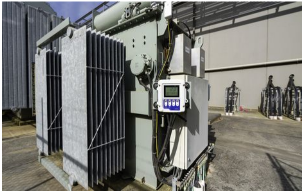
The B100 installed on a distribution transformer, calculating the hot spot and the ageing of the insulating paper in real time.
