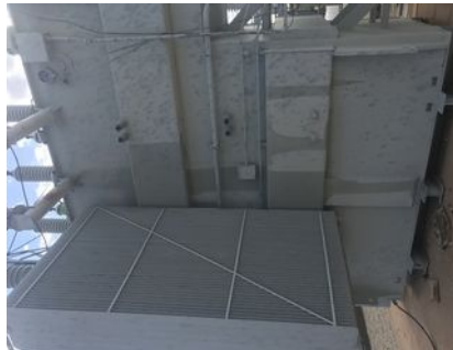
Cooling radiator, with the fans and pumps monitored by the unit.
